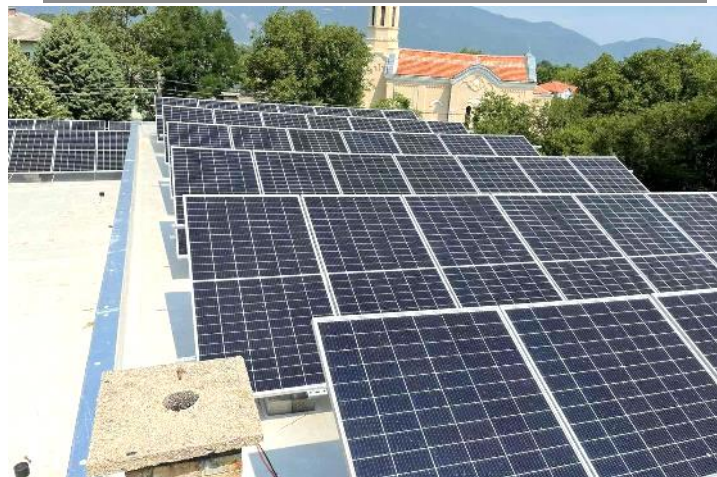
Installation of solar panels on rooftops of public buildings in the municipality of Maglizh
